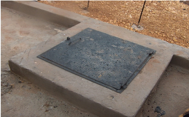
Photo 9: Sludge Holding Tank
