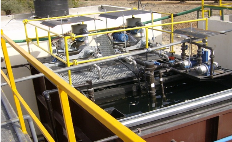
Photo 6: Activated Sludge System (AS)
