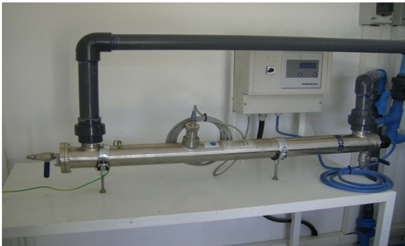
Photo 11: UV Disinfection Unit
