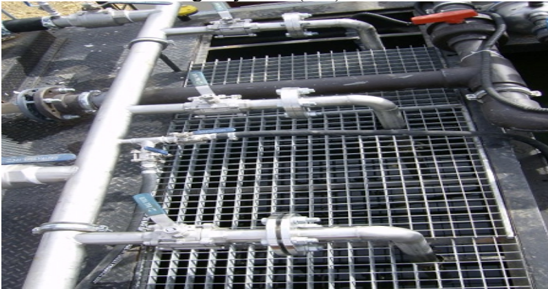
Photo 7: Aeration Tank and Air Blowers
