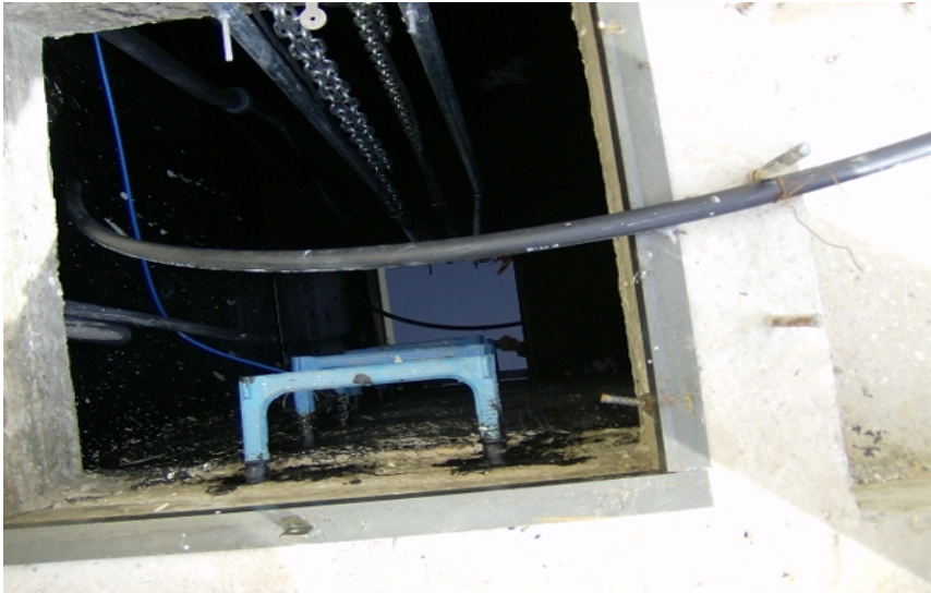
Photo 2: Pit Station and Lifting Pumps
