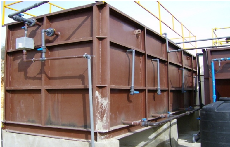
Photo 5: Anaerobic Baffled Reactor (ABR) Compartments
